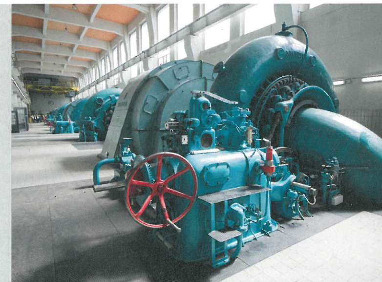
The stoRE project focuses on pumped storage plants like this turbine in Waldeck, Germany.
